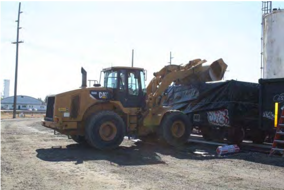
Loading waste from Pond C into lined railcar for transport to waste disposal facility.
