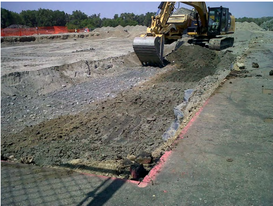
Pond A – Removal of 2 to 4 foot bgs layer under top liner. Facing northwest.
