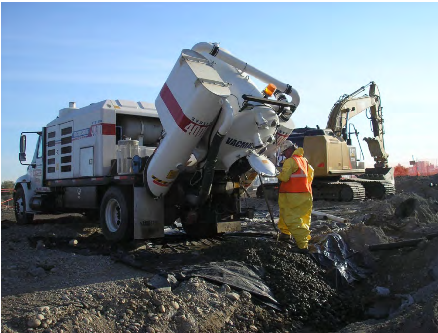
Soil cuttings from Pond C test pit C-6 being dumped onto visqueen to allow sample collection.
