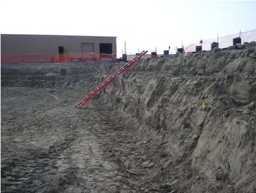
Pond B – West wall following excavation. Flagging shows sample locations. Facing South.
