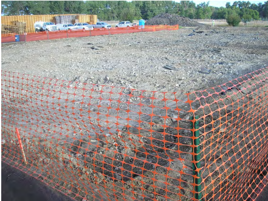
Pond B – Following removal of overburden above the top liner. Facing northwest.
