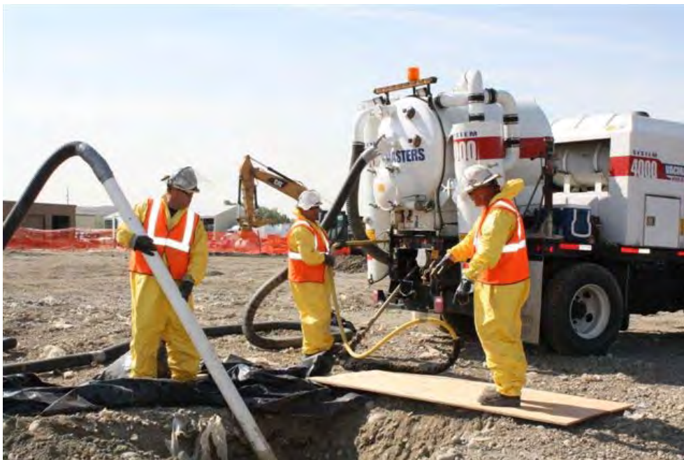
Pond C – Potholing in test pit to locate depth of bottom liner.
